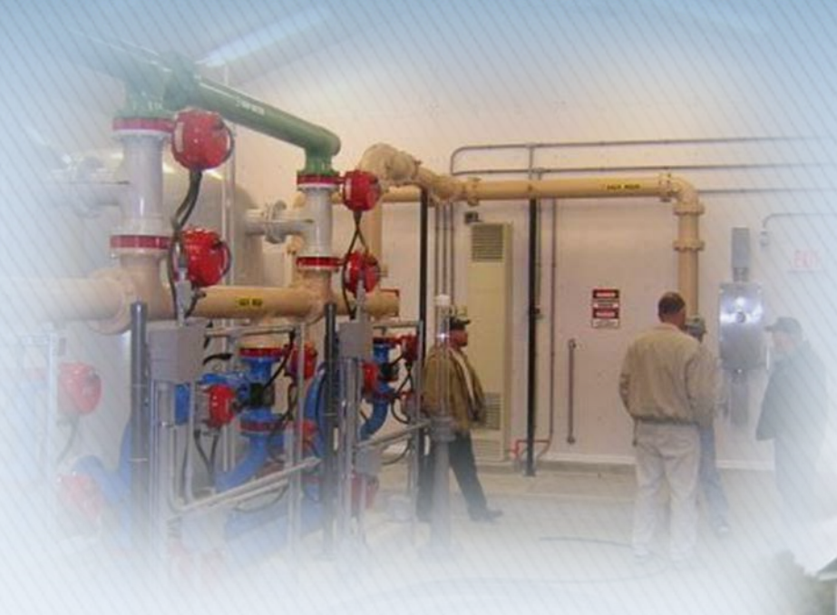
Manganese Removal Filters
