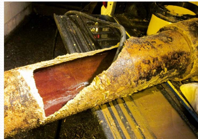
This is a typical water main break in an 8 inch concrete pipe. This section was removed from a break on Washington Street in October 2011.
